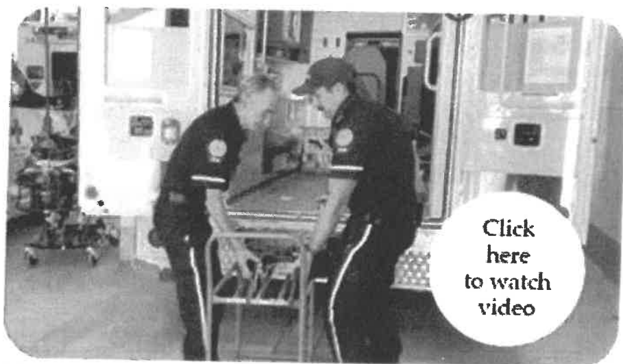
EMS technicians work to install power lifts in one of 10 additional new ambulances. There is a commissioning period required before new ambulances are ready to join the fleet.
